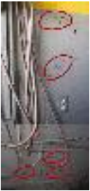
Water marks of all the flooding
